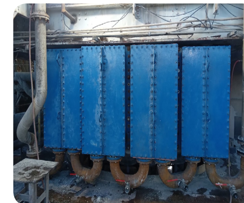
The newly installed tube bundles
